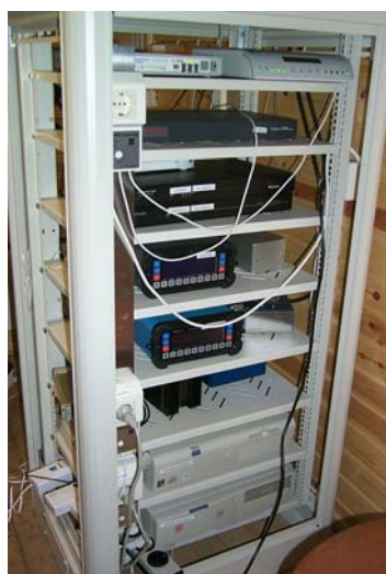
Figure 3: Interior of a SWEPOS station.
