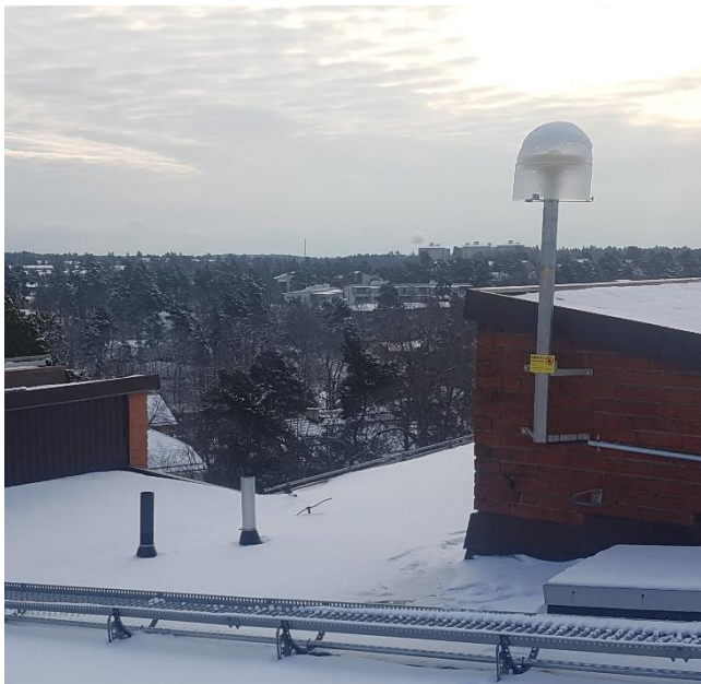
Figure 4: Gustavsberg is a SWEPOS class B station with a roof-mounted GNSS antenna mainly established for network RTK purposes.
